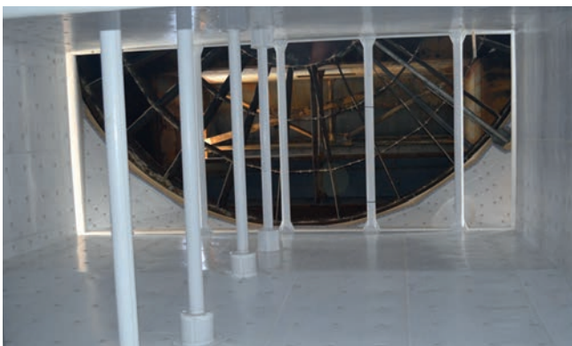
PFA lining in a raw gas duct
