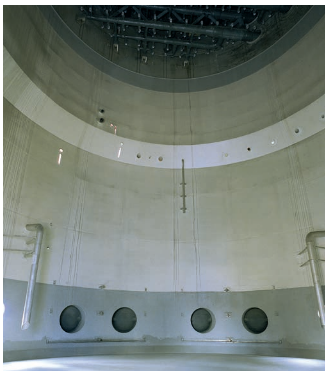
Lined flue gas scrubber
