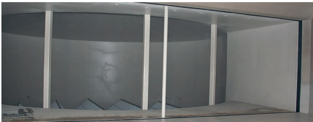
Coated clean gas duct
