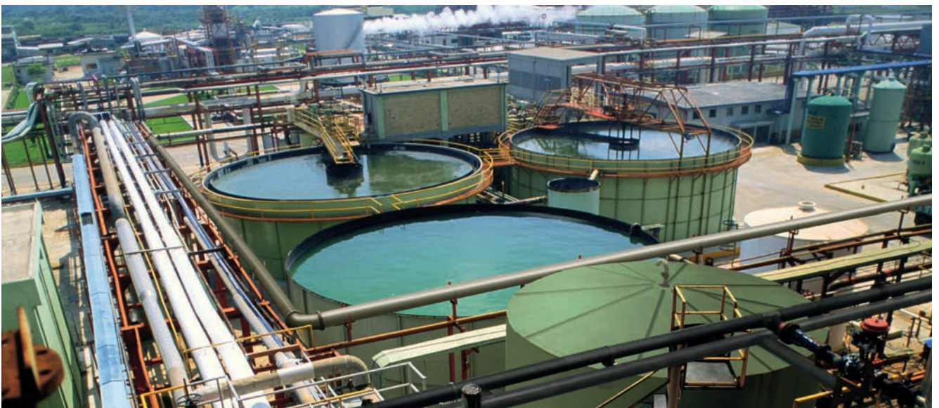
Rubber-lined sedimentation tank
